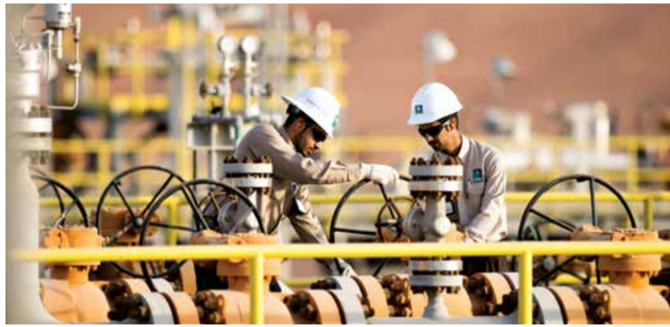
A core element of Saudi Aramco's Safety Management System focuses on asset integrity, which describes the life cycle management processes for the integrity of the company's varied assets.
