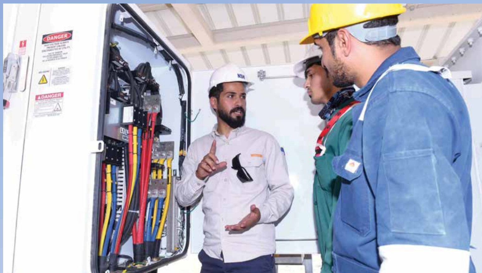
From left, Wayil AlAnezi, Hussain Albu Hassan (NSH), and Ali AlAmer, are some of the technicians with the crew who installed the devices that direct power to the equipment within the oil well infrastructure. The crew composed of 78 Saudis completed all the necessary work for building ABHD-131, ranging from project management, and quality assurance to actual site execution such as welding and instrumentation.
