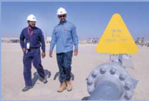
Left, Khalid M. Al Shammari, quality control engineer of the crew, and Abdullah Albuaynian, planning engineer of the crew, make inspection rounds on the flow lines. The Saudi crew met the quality requirements and completed the work safely and ahead of schedule due to the detailed planning, diligent execution, and teamwork spirit.
