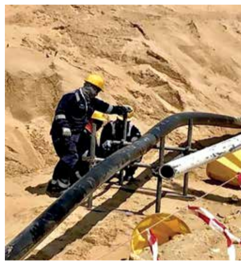
Crews deploy reinforced thermoplastic pipe (RTP) in Khursaniyah. A well-proven technology that has proven to be a vital product for Saudi Aramco's oil production facilities, the use of RTP is just one of the many nonmetallic solutions being applied by the Manifa Producing Department, and across the company as a whole.
