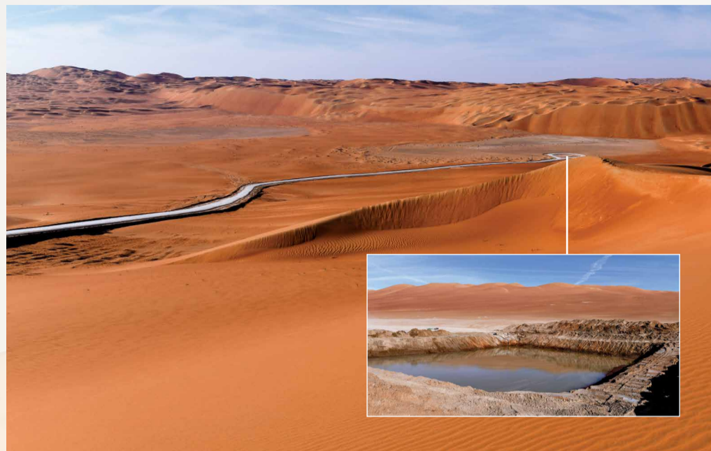
A meandering 16-km road, with a base built from local sabkha material, will take visitors in buses and light vehicles on an immersive journey to three visitor viewpoints, and through the inner area's six salt flats. Past a natural oasis formed by ancient salty water lying three meters below the surface, visitors will see the tough Tamarix aphylla (salt cedar) trees that with their deep taproot systems, provide shade and contribute to the area's growing biodiversity restoration.
