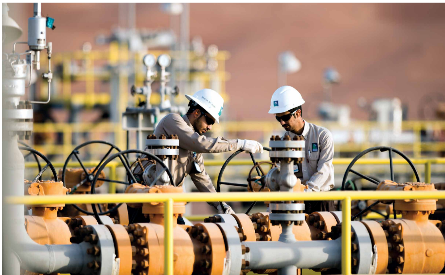
Turnaround and inspection ensure critical inspection and maintenance work is carried out for continued safe operations. Since the introduction of a specific unit to assist in performing the critical function, Aramco has seen a marked improvement in turnaround safety performance across the whole of the company, resulting in zero significant incidents or injuries.
