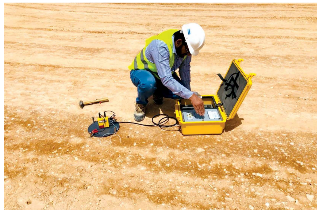
Saudi Aramco recently introduced the use of electrical density gauge technology to measure the density of compacted soil at construction sites on the Ajyal project. Deployment of the relatively new compaction measurement technology is not only safer than other commonly used technologies; it's less expensive, too.
