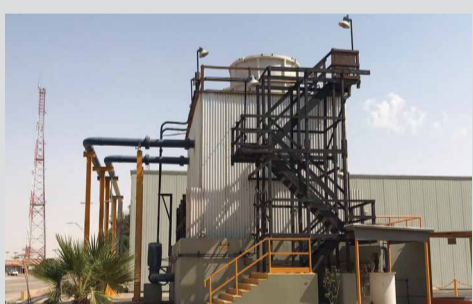
Water is a particularly treasured resource in Saudi Arabia, and the Abqaiq air-conditioning plant cooling tower uses tertiary treated sewage effluent instead of non-replenished raw water.
