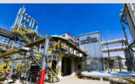
Rather than sending CO 2 to a stack, an internally geared compressor at the Hawiyah NGL recovery plant uses seven stages to compress CO 2 , where the fifth stage involves routing to a gas dehydration unit, before being returned for stages six and seven in the compressor.
