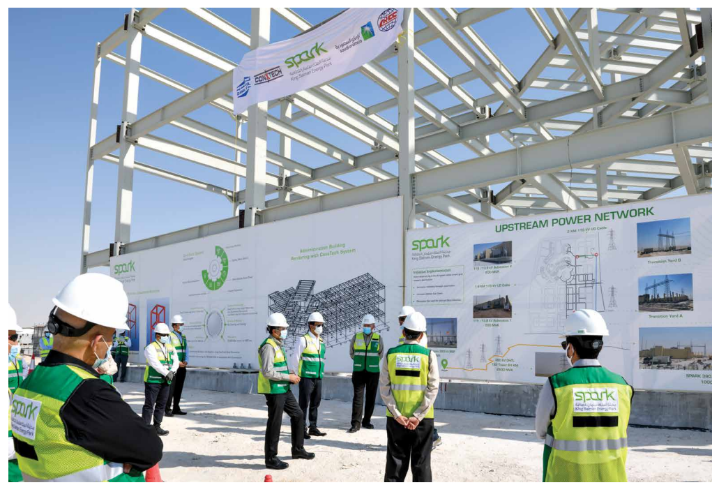
Site exhibition of first ConXtech building to Aramco senior management at the SPARK project.
