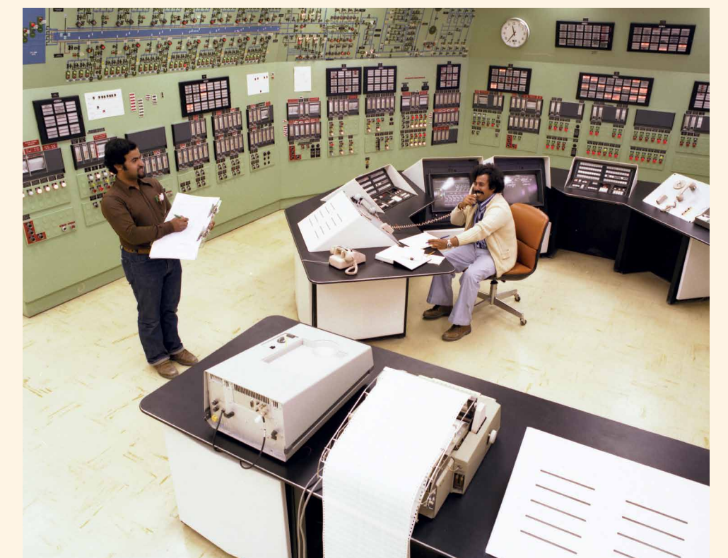
Operators in the control room of the Qurayyah Seawater Treatment Plant in 1979 monitor the processing and delivery of 4.2 million barrels per day of seawater for injection into oil fields to maintain reservoir pressure.
