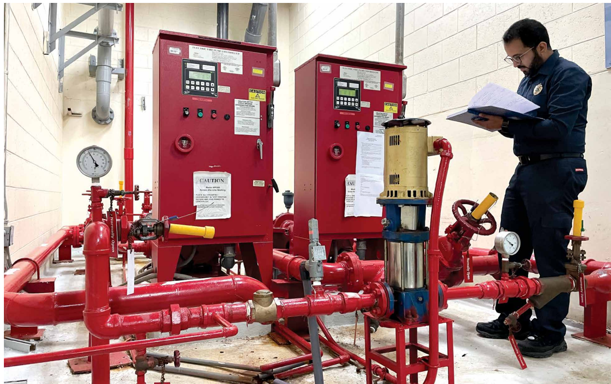
An inspector records the fire water pump data during an annual pump performance test.
