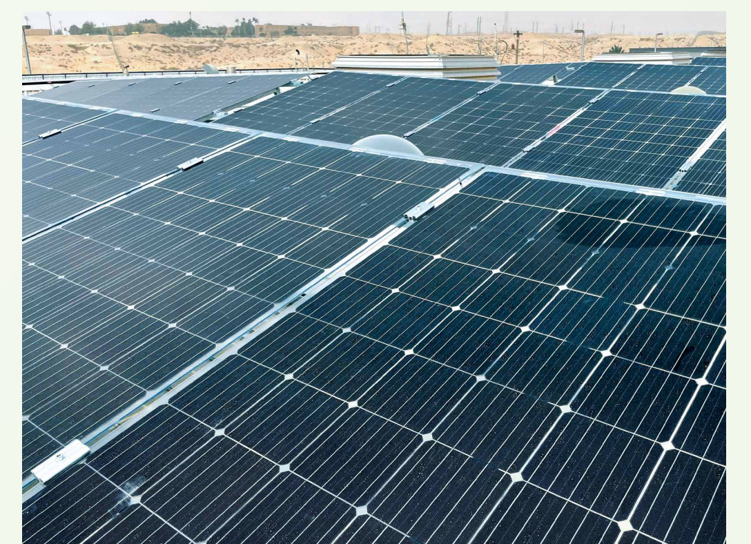
The South Ghawar Producing Department expects a solar powered air-conditioning system introduced in November 2020 to its ‘Udhailiyah office and maintenance building to deliver up to 45% energy savings.
