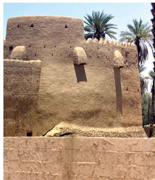
Certain parts of Ibn Rumman Palace were built 170 years ago. While the interior is not open to visitors, people can admire the craftsmanship of the external wall and towers.
