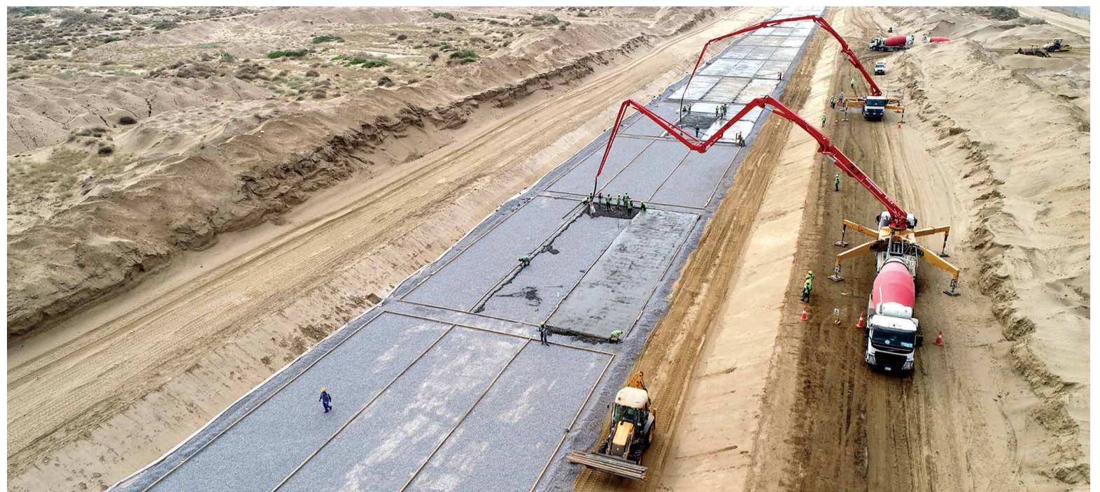
Nonmetallic solutions have been deployed successfully at Jazan operations, including using glass fiber reinforced polymers bars for a 20-km concrete flood mitigation channel.
