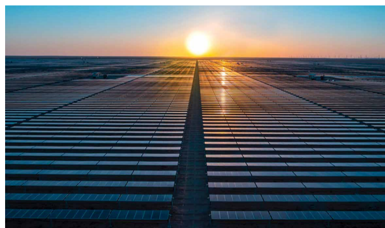
Aramco's 30% investment in the Sudair Solar PV project reflects the company's efforts to advancing sustainable energy solutions within its operations.
