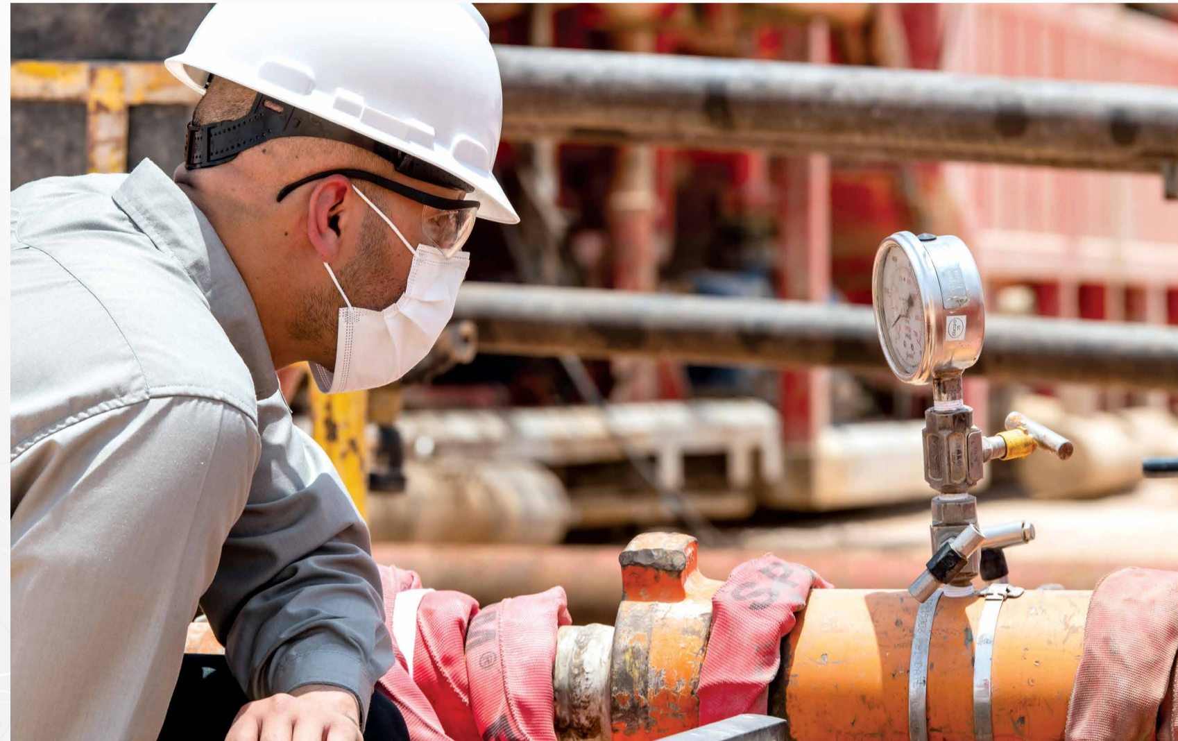
Foreman Saad S. Garni monitors the successful connection of a gas tie-in from drilling rig ADC-45 to the wellsite's production manifold flow line.
