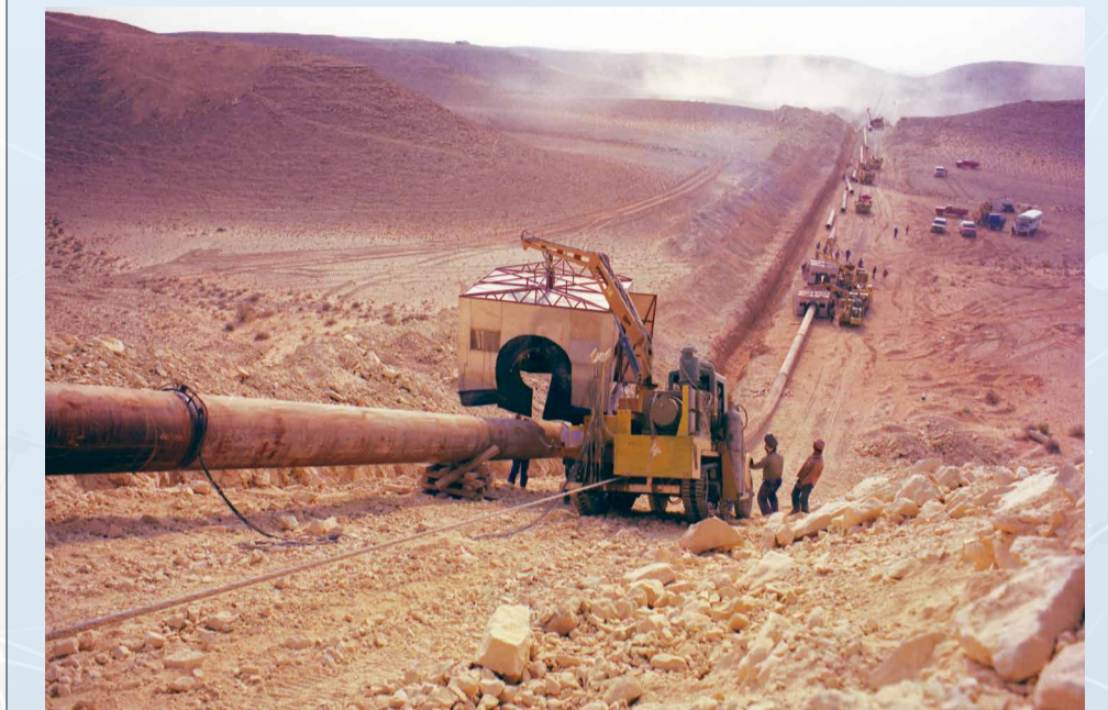
A 1,170-kilometer NGL pipeline links Yanbu' and Shedgum.
