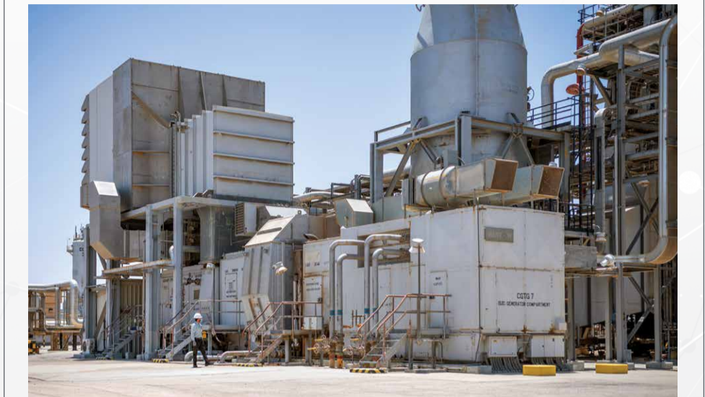
Abqaiq Plants cogeneration system.
