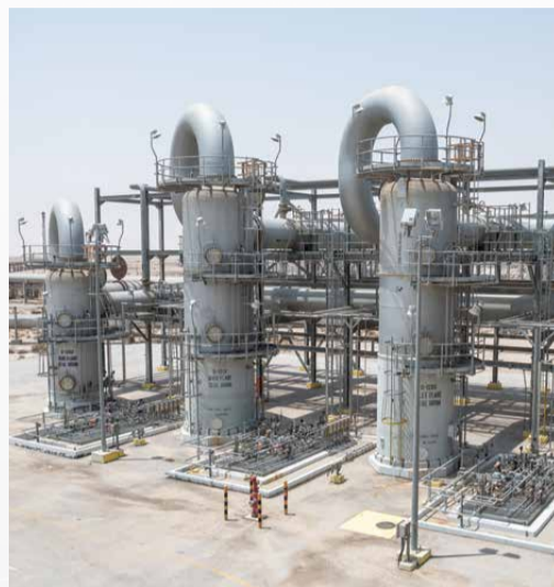
This flare gas recovery system in Shedgum helps prevent gas from being flared on a regular basis.
