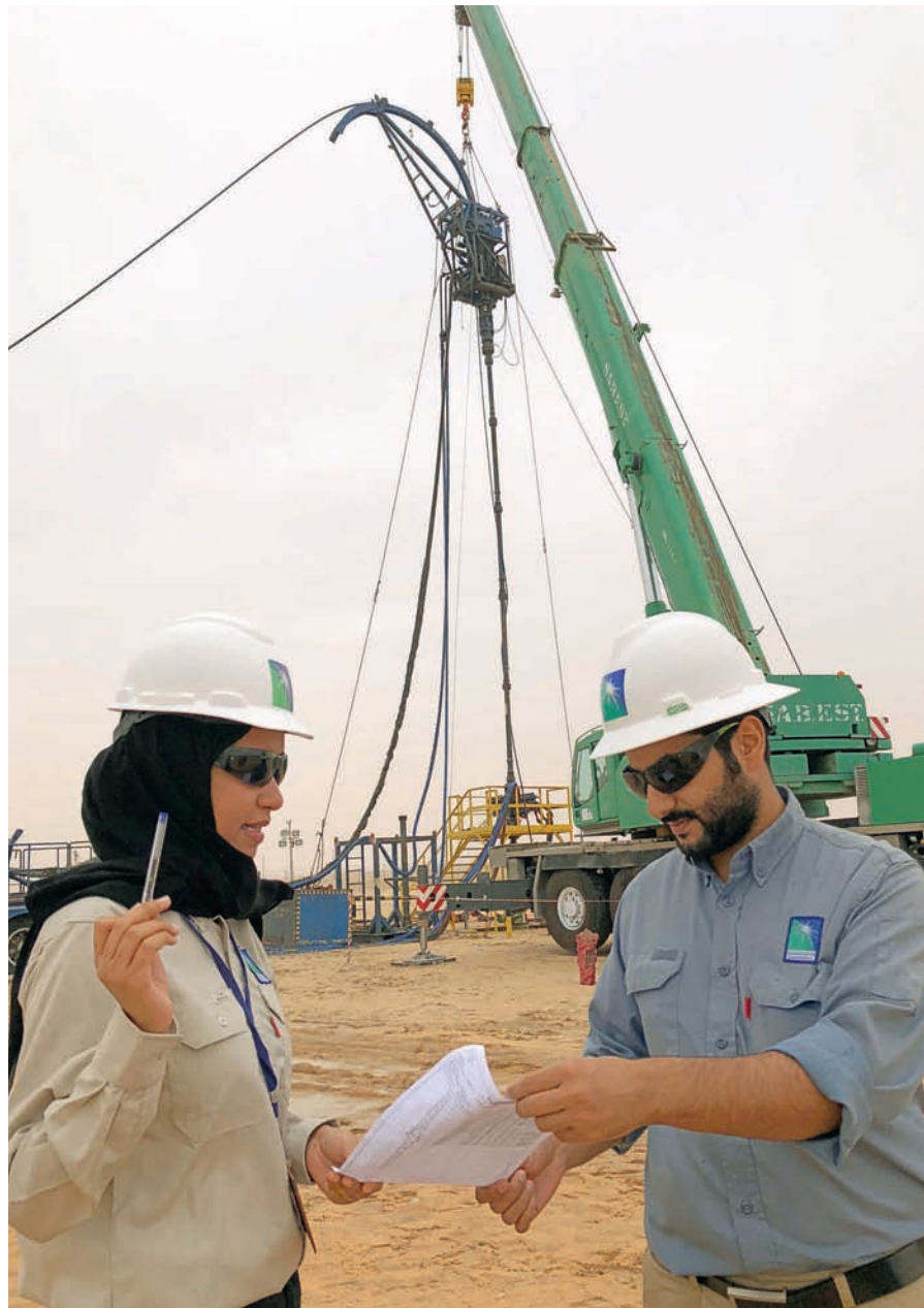
Fatimah Alkayadi in discussion with the site foreman about the logging procedure making sure the objective of the operation is accomplished.
