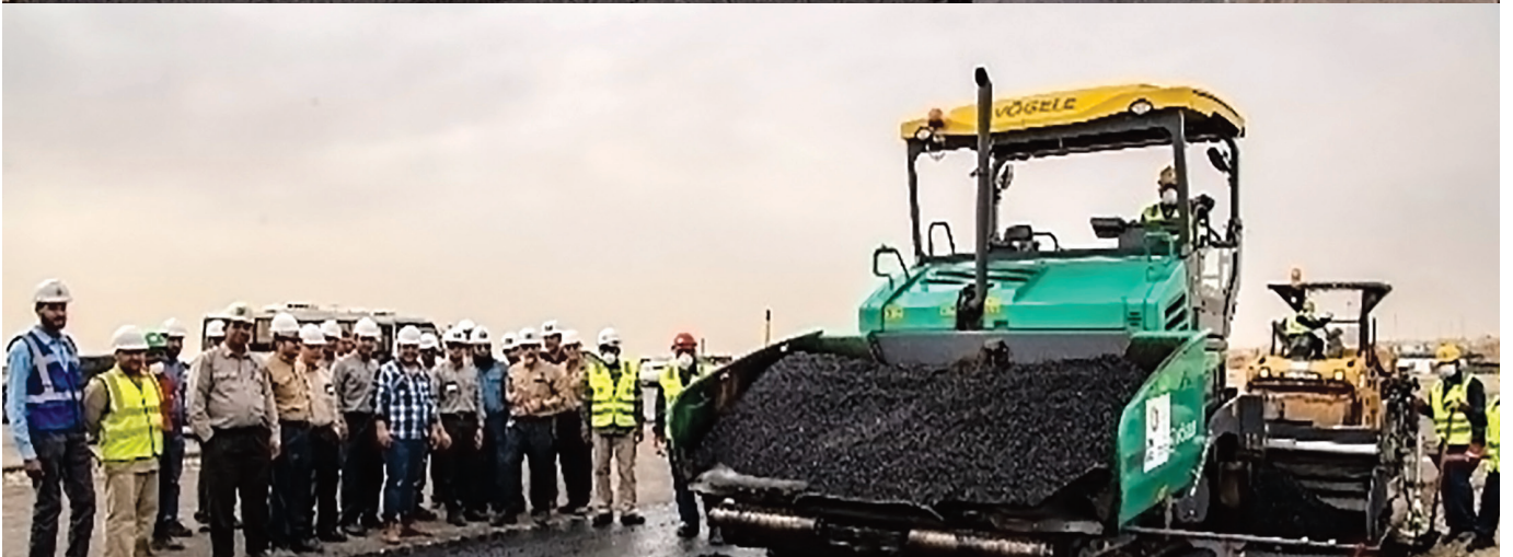
The above photographs show the innovative concept of turning crumb rubber from tires into a form of asphalt used in laying and maintaining roads, such as the road construction project at North Jiddah Bulk Plant Expansion Project
