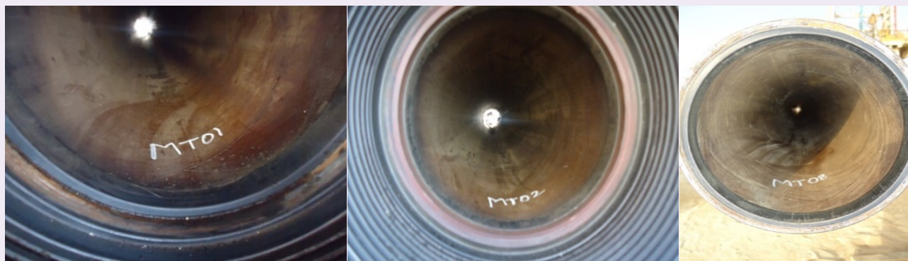
Fig. 5 GRE lined tubing that was pulled out from a water supply, Well-2.
