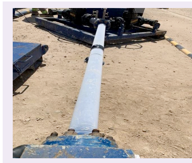
Fig. 7 Ice formed on the pipeline, indicating the formation of gas hydrate.
