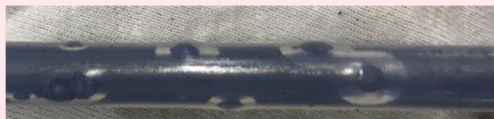
Fig. 5 The Cu_2S bumps growing under the PFA cable insulation inside a penetrator capillary tube.
