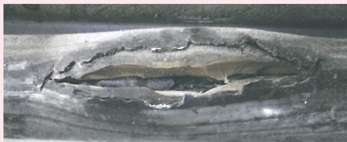
Fig. 4 A burst in a penetrator tube due to excessive pressure exerted by the growth of the copper corrosion byproduct.
