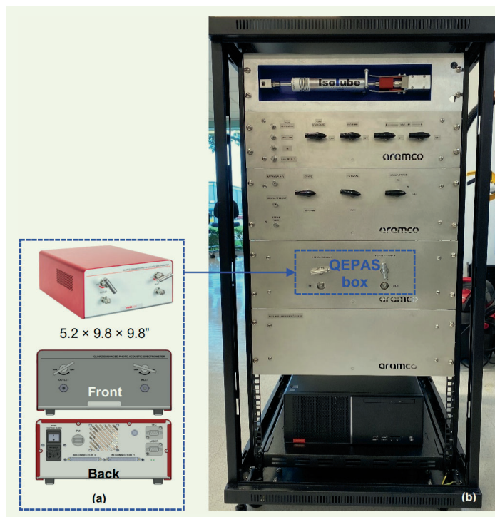
Fig. 2 The realization of a QEPAS-based gas analysis system: (a) The portable QEPAS sensor box, and (b) All the components of the QEPAS assembled in a rack.
