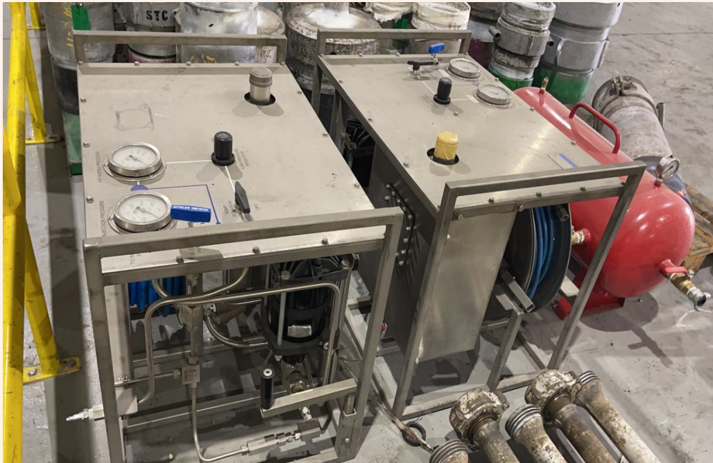
Fig. 3 An image of the high-pressure, low rate pumps.
