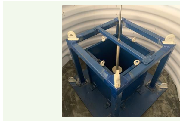
Fig. 8 A large block mold inside the curing tank ready for pouring the cement grout. The wax structure is installed to cast the borehole with a weak point (shown here by U-shape circular notch).
